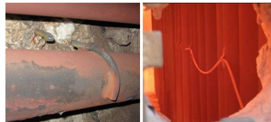
ABOVE LEFT: Severed TSTC due to unrealized heat expansion. ABOVE RIGHT: Improper routing of TSTC may appear correct at time of installation but unreliable during operation.
